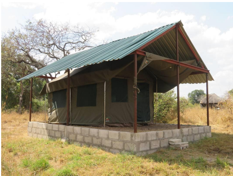
Fig. 4 – A new tent and platform at Kafue camp for lodging new Junior Field Ecologist Moses Muwowo. The platform is necessary to keep the tent out of water during the wet season and the roof helps keep the tent cool as temperatures soar in the hot dry season.
